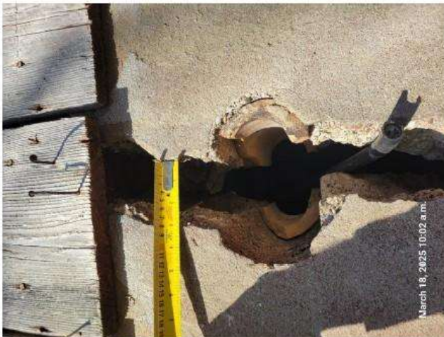
Severe crack in concrete foundation
